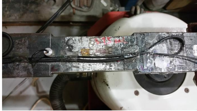
Figure 1. Damage in the steel beam
