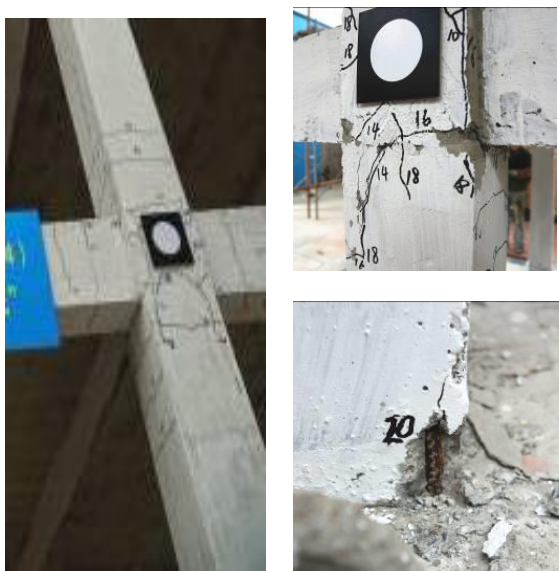
Figure 4.1 Failure mode of RCF model
