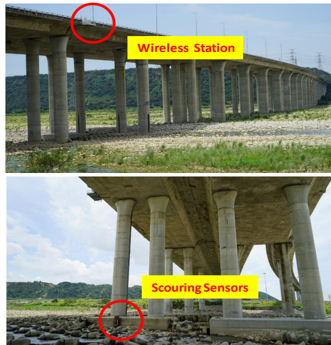
Fig. 2 Scouring sensor field deployed
