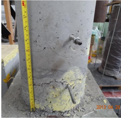
Figure 4.5 The photo of the crack at the plastic hinge zone.
