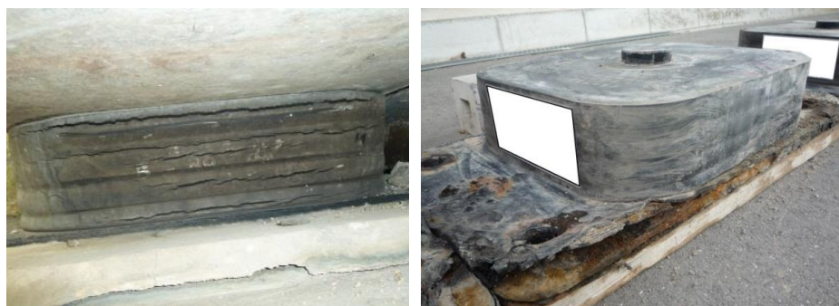
Figure 2.2 Damage status and cracks of ring bearings
