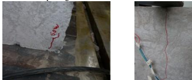
(c) horizontal crack and spalling at bottom (d) vertical crack at contact surface
