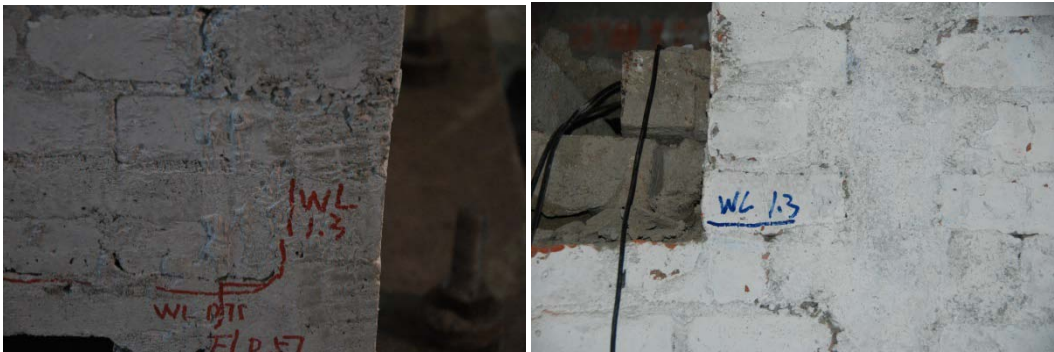
a Diagonal crack at the corner of window in axis ① b Diagonal crack at the corner of window in axis ② Figure 4.3 Destruction of model F
