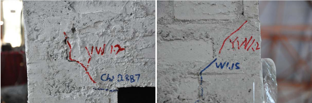
a Diagonal crack at the corner of window in axis ① b Diagonal crack at the corner of window in axis ② Figure 4.2 Destruction of model E
