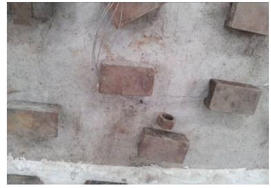
Figure 2.7 The surface of slab after fire
