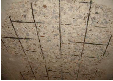
Figure 2.6 The bottom of slab after fire
